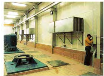
Varitone® sound-absorptive wall linings for a water pumping station
