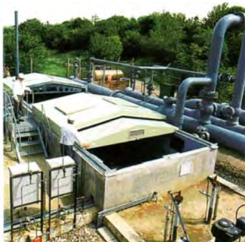
Sliding acoustic pit covers for a British Gas regulator station.
