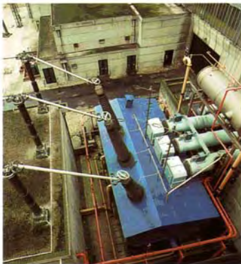
One of 7 Moduline® acoustic enclosures controlling generator transformer noise emissions at Didcot Power Station (UK).
