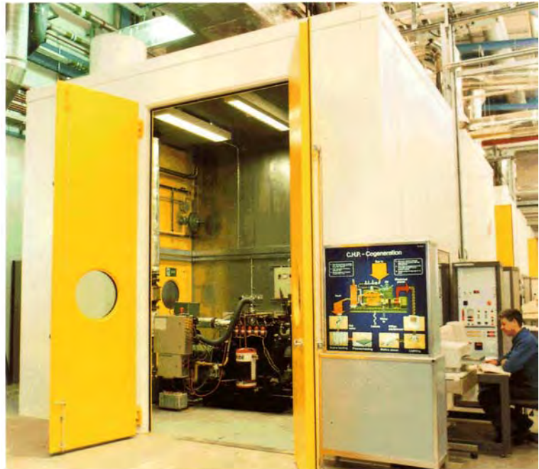
Large Moduline® engine test cells for British Gas.
